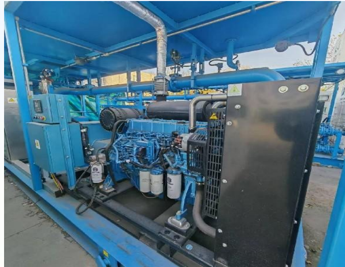
Booster Pump skid
