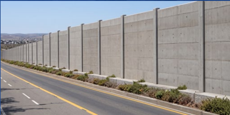
① Flood wall (3.6km-long, 2m-high)
