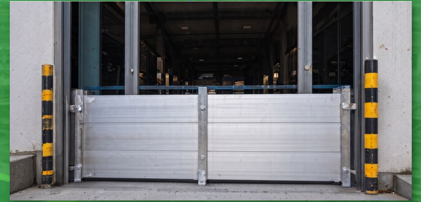
③ Flood gates at plant entrance
