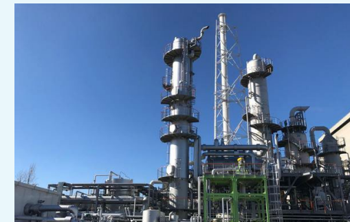
Commercialized plant No.2 (Sumitomo Joint Electric Power Co., Ltd)
