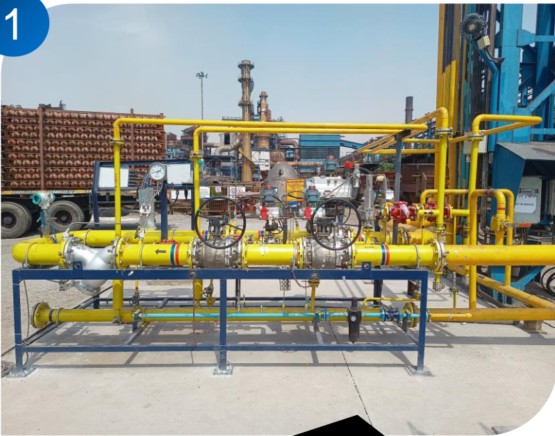
Valve station-1 Reduction of pressure: 200-5 bar(g)
