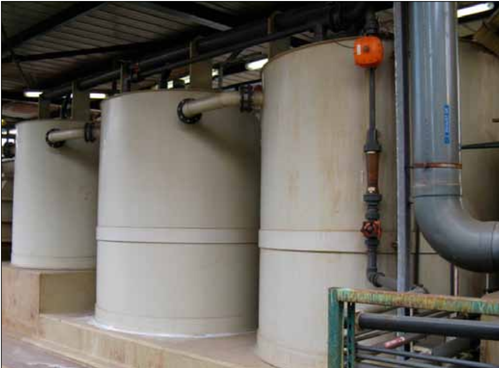
Figure 7.1.2 The two neutralisation tanks and the flocculation tank
