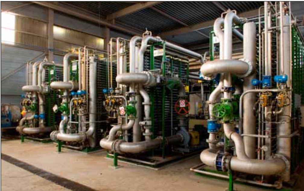
Figure 7.2.2 The four ultrafiltration skids
