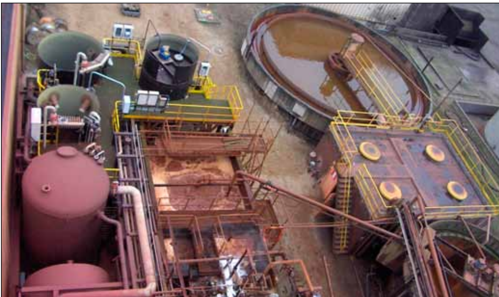
Figure 7.2.1 Overview of the physical-chemical treatment plant of the pickling lines
