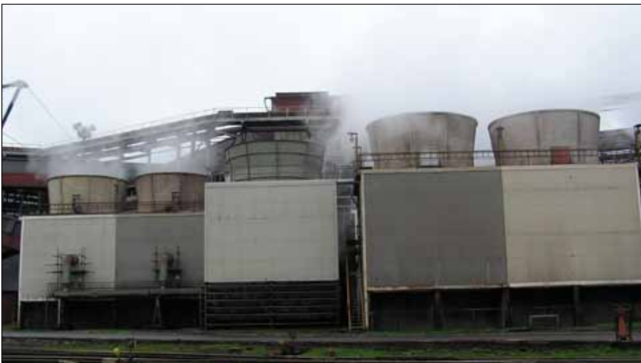
Figure 5.2.1 BOF water treatment system cooling towers
